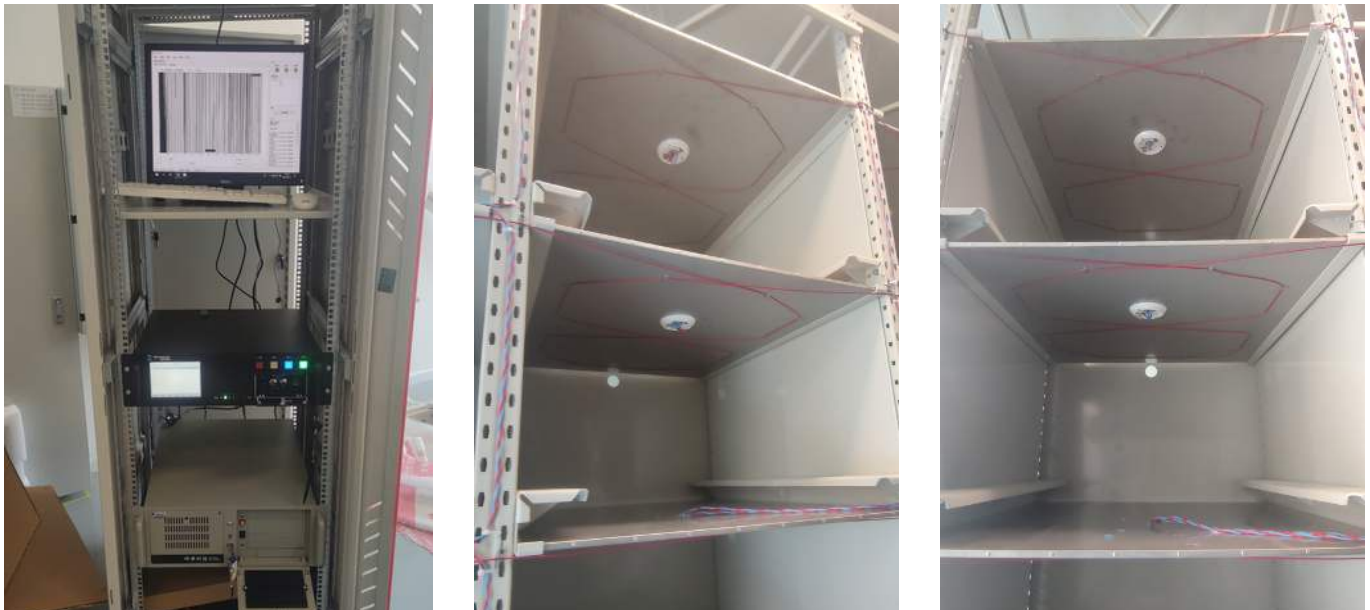
Figure 3: Sensing cable set up throughout storage bays with single FireLaser unit
